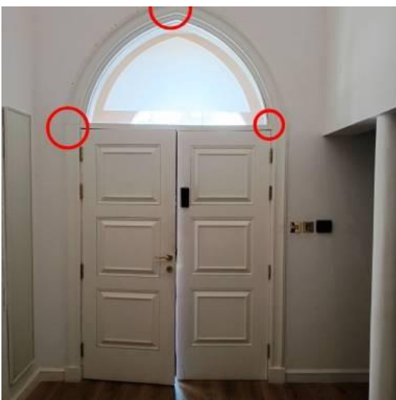
Created: Sat 22 Nov 12:16 2025 Location: Entrance Status: open Comments: Sealant missing in door frame joints
