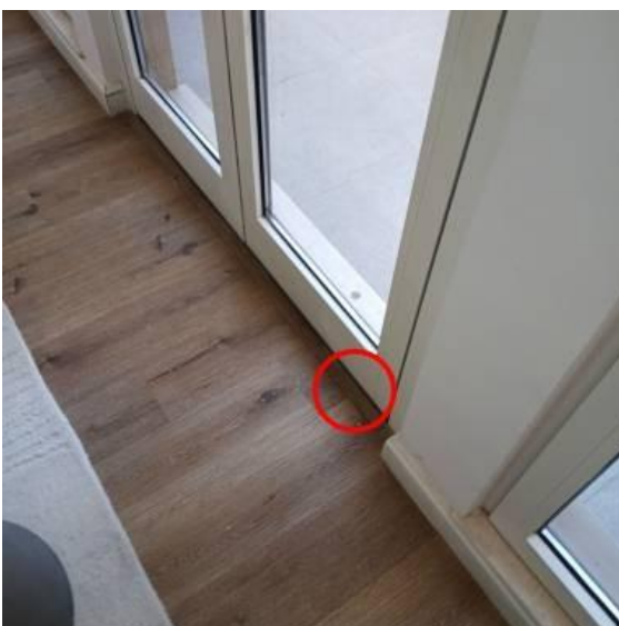
location: Dinning Room Status: Open Comments:
