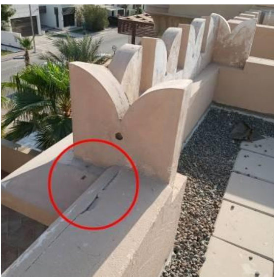
location: Roof top Status: Open Comments: Damaged were noted on parapet wall
