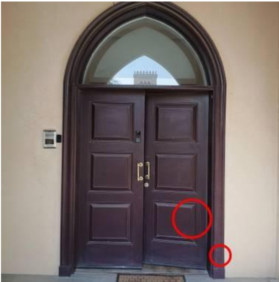
Created: Sat 22 Nov 12:13 2025 Location: Entrance Status: open Comments: Multiple cracks on door and door frame
