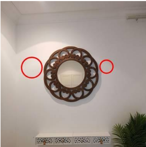
location: G.F Bedroom 1 Status: Open Comments:
