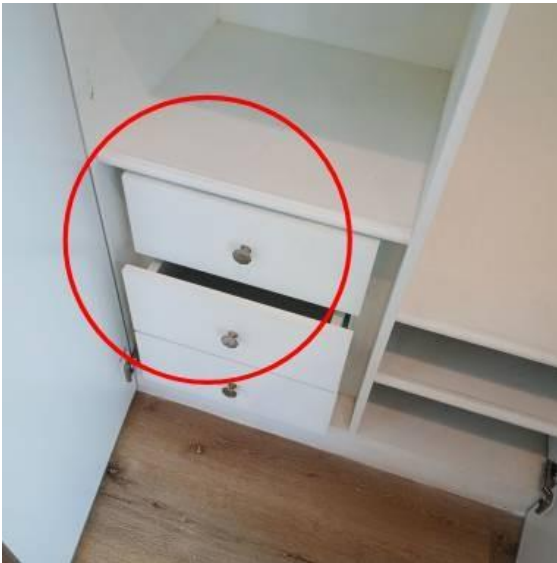
location: 1st floor Bedroom 3 Status: Open Comments:
