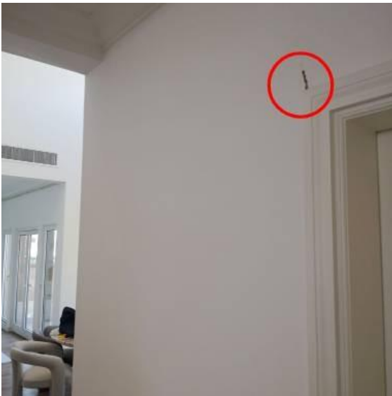
location: Dinning Room Status: Open Comments:
