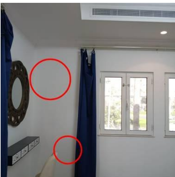
location: 1st floor Bedroom 3 Status: Open Comments:
