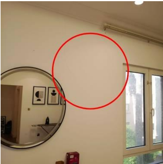
location: 1st floor Bedroom 4 Status: Open Comments:
