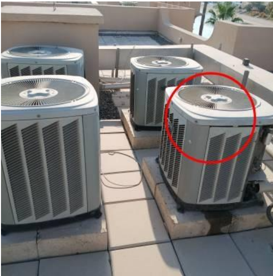
location: Roof top Status: Open Comments: Found Noisy outdoor AC unit
