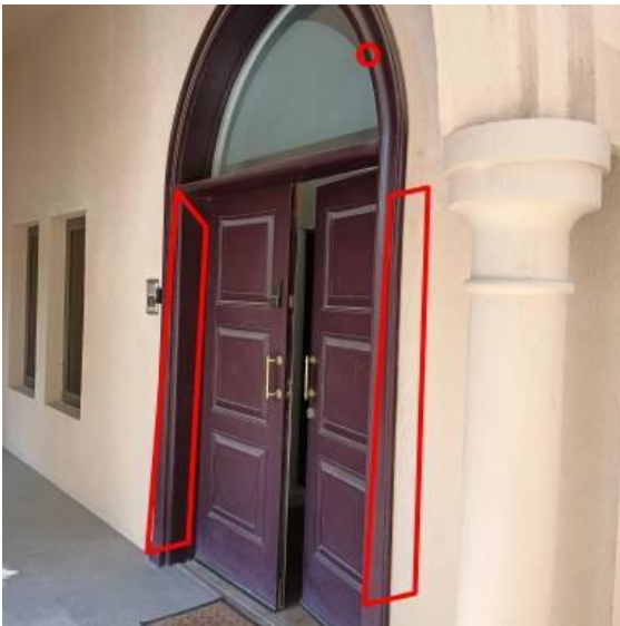
Created: Sat 22 Nov 12:15 2025 Location: Entrance Status: open Comments: Multiple cracks and chipped on door frame
