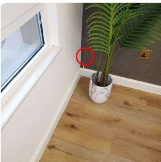
location: 1st floor Bedroom 4 Status: Open Comments:
