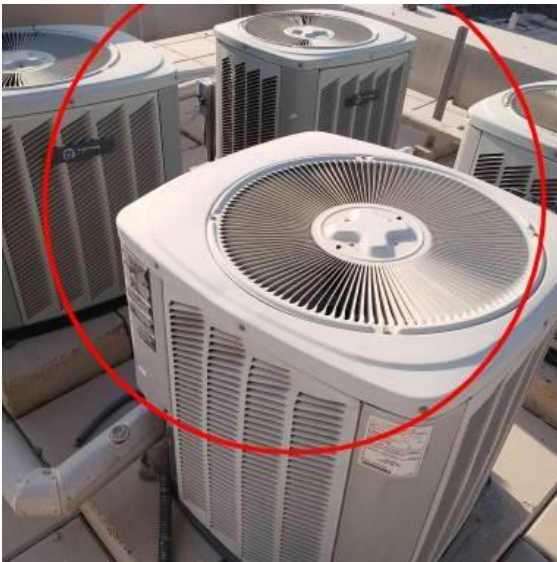
location: Roof top Status: Open Comments: All outdoor AC unit requires cleaning
