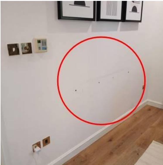
location: G.F Bedroom 1 Status: Open Comments:
